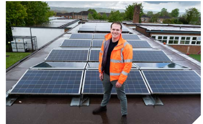
Rose Hill Primary School Solar PV array
